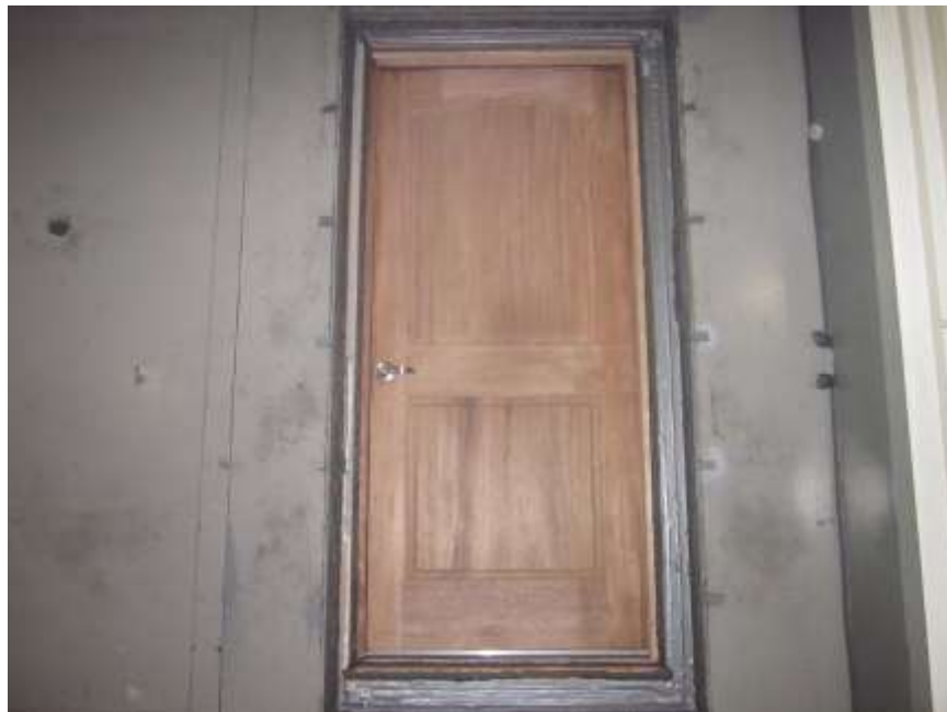
Source Room View of Installed Test Option A
